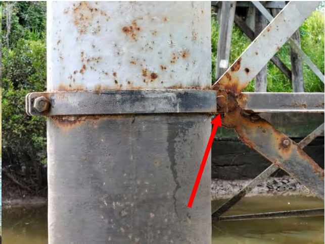
Photo 16 Pier 5 corrosion on bracing element fixings
