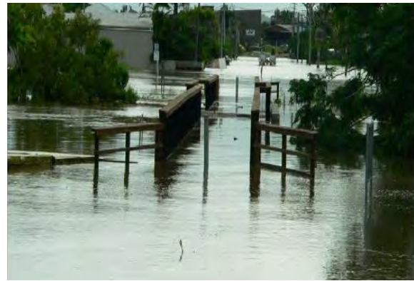
Figure 12: 2010 flood, showing water over the bridge decking (Picture Bundaberg, Ref#02403).
