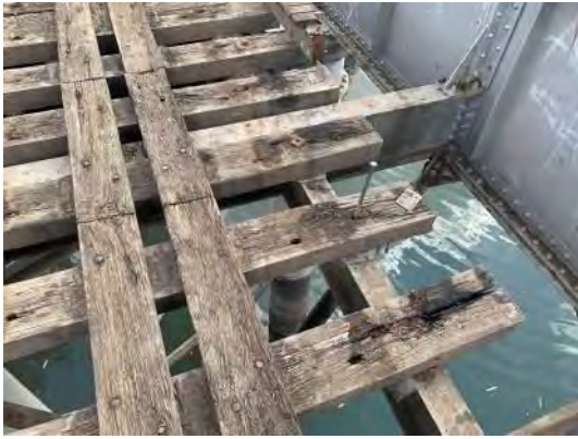
Figure 52: Badly deteriorated timber sleepers (Bligh Tanner 2022).
