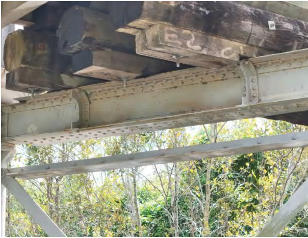
Photo 37 General view pier 6 cross beam, isolated areas of surface corrosion
