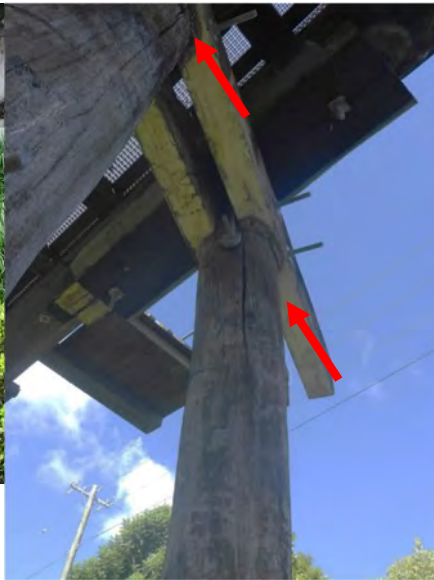
Photo 24 Pier 7 vertical splitting below headstock
