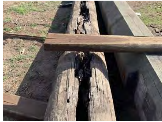
Figure 53: Badly deteriorated girder (Bligh Tanner 2022).
