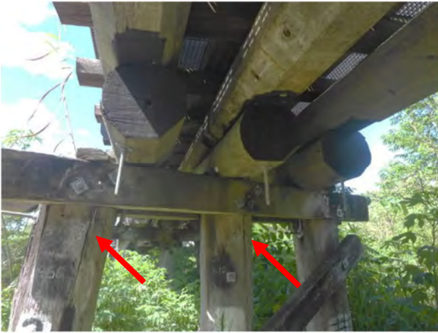
Photo 5 Pier 2 vertical splitting
