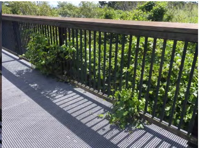
Photo 81 Excessive vegetation on left hand side railing near approach 2
