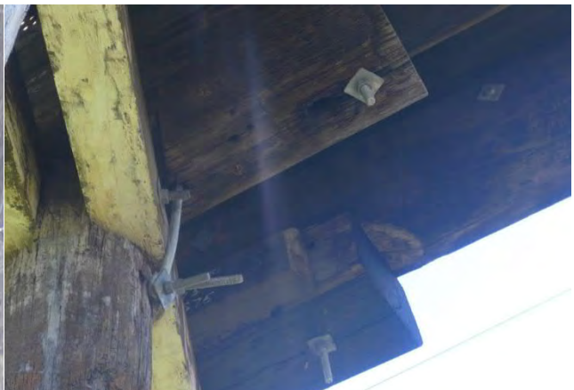
Photo 26 Pier 7 tie rod on abutment 1 face bent
