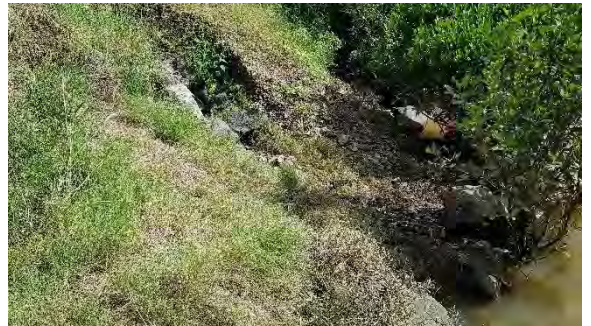
Figure 71: Erosion on the NW river bank (Converge 2022).
