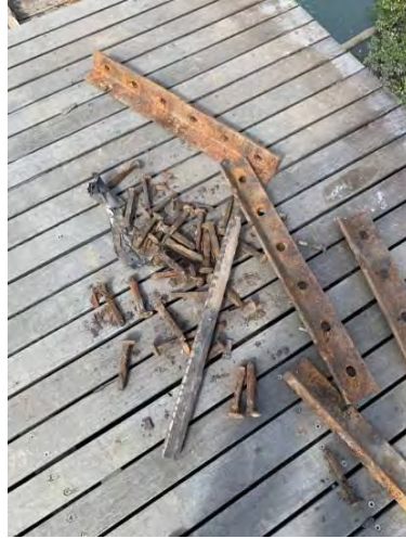
Figure 50: Heavily corroded bolts and steel connections (Bligh Tanner 2022).
