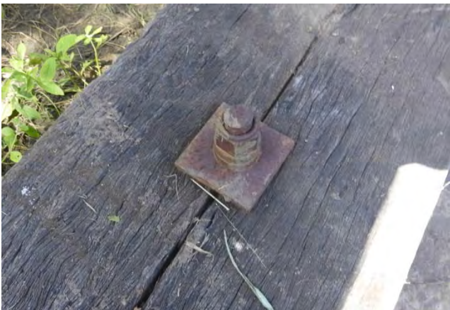
Photo 25 Pier 7 timber footing bolts exhibiting surface corrosion
