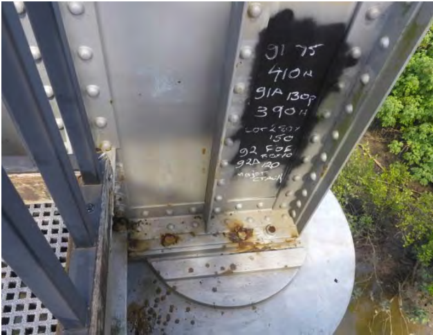
Photo 65 Main girder to bearing plate bolts corrosion
