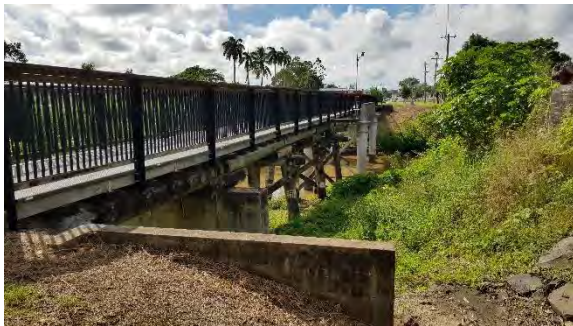
Figure 76: View east along south side of bridge; note overgrown embankment and short retaining wall (Converge 2022).
