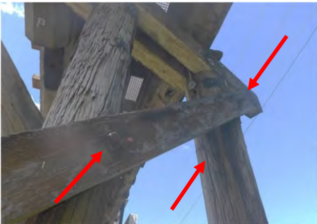
Photo 11 Pier 4 cross bracing bolts surface corrosion, vertical splitting in piers
