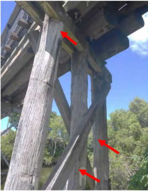
Photo 9 Pier 4 vertical splitting
