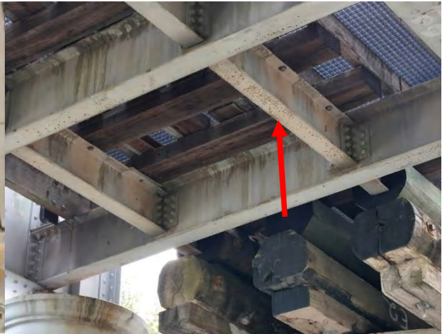
Photo 58 Span 6 strut beams surface corrosion
