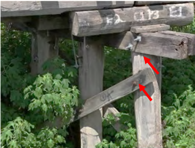
Photo 7 Pier 3 cross bracing bolts surface corrosion, vertical splitting below headstock
