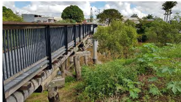
Figure 77: View west along north side of bridge, note the overgrown embankment (Converge 2022).
