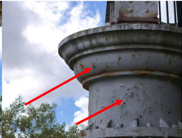
Photo 68 Bearing plate corrosion spots
