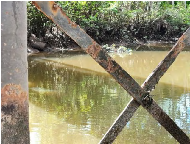
Photo 15 Pier 5 corrosion on bracing elements
