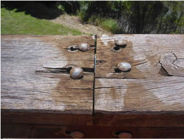
Photo 78 Top railing fixings installed incorrectly
