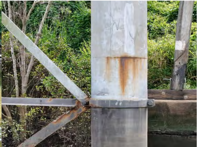
Photo 22 Pier 6 corrosion staining at welds in tidal zone
