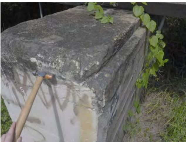
Photo 3 Pier 1 side 1 concrete delamination, 300 mm x 200 mm
