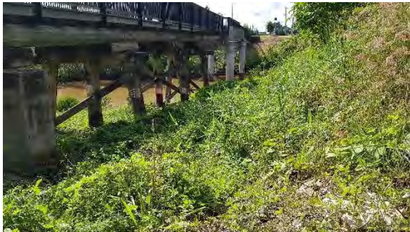
Figure 70: Overgrown area on the SW side with erosion noticed caused by water from a drain up top (Converge 2022).
