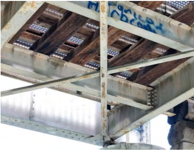
Photo 59 Span 6 cross bracing surface corrosion
