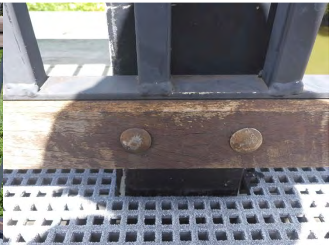
Photo 77 Bridge railing fixings surface corrosion
