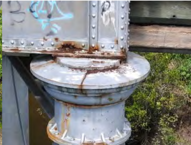
Photo 66 Bearing plate surface and crevice corrosion
