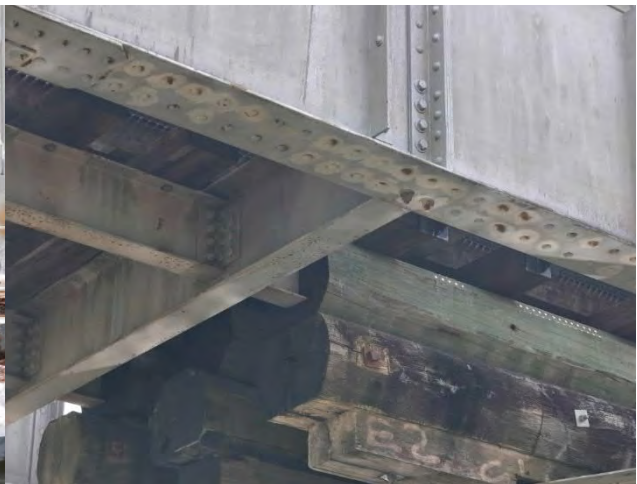
Photo 56 Span 6 main girder bottom flange rivets surface corrosion
