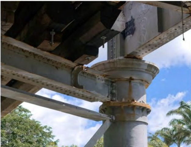
Photo 67 Bearing plate corrosion staining
