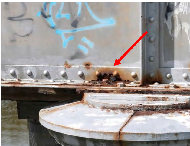
Photo 55 Span 6 main girder left hand side web corrosion
