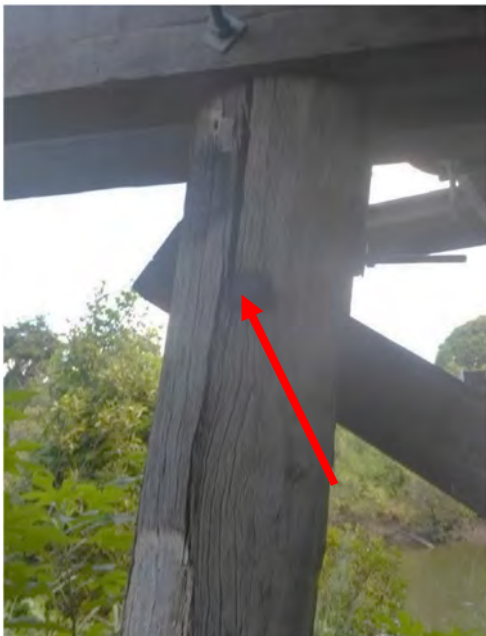
Photo 29 Pier 8 timber splitting, cross bracing bolts exhibiting surface corrosion
