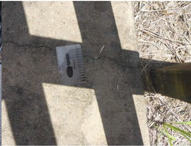
Photo 72 Cracks up to 0.3 mm in approach 2 footway slab
