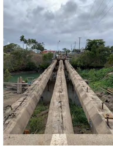
Figure 51: View from Span 1 to 5, almost all girders badly deteriorated (Bligh Tanner 2022).
