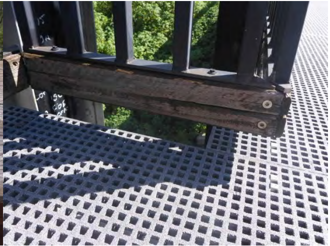
Photo 79 Timber splitting at toe boards
