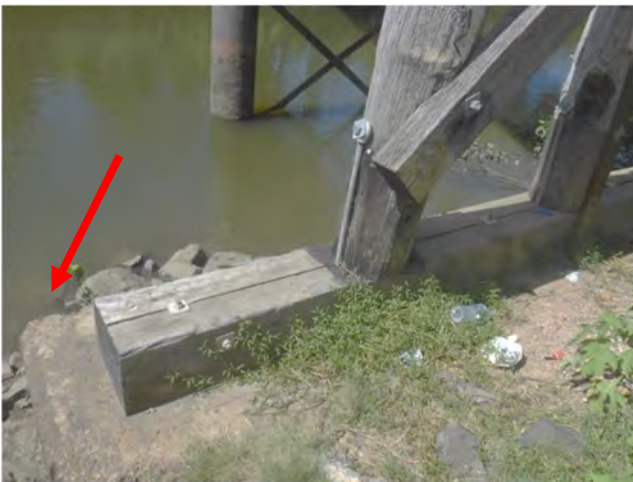
Photo 13 Pier 4 footing corner spall, 300 mm x 300 mm
