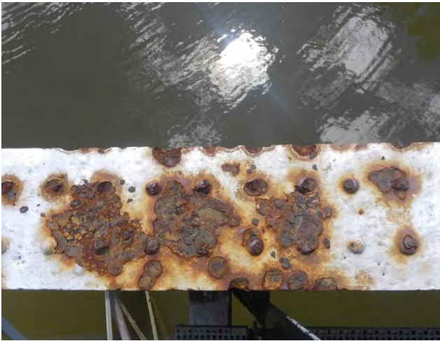
Photo 53 Span 6 main girder pitting corrosion
