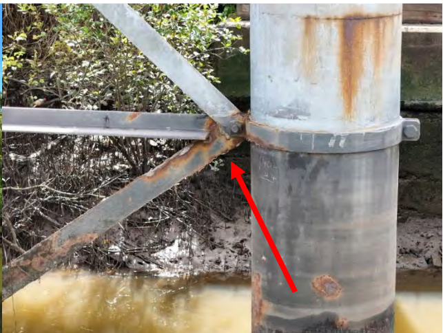
Photo 20 Pier 6 corrosion on bracing elements
