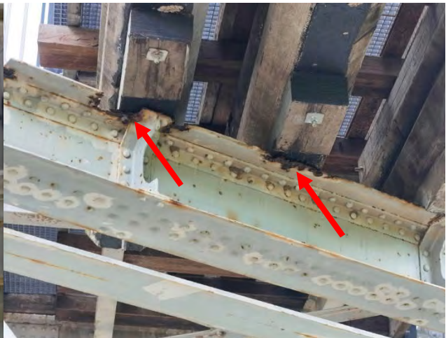
Photo 36 Pier 5 cross beam top flange section loss
