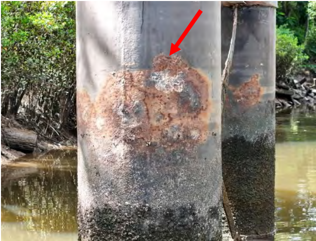
Photo 21 Pier 6 surface corrosion and pitting corrosion in tidal zone
