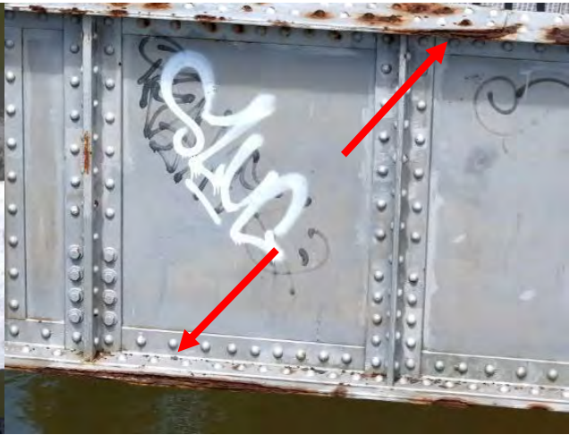
Photo 54 Span 6 main girder left hand side flange corrosion
