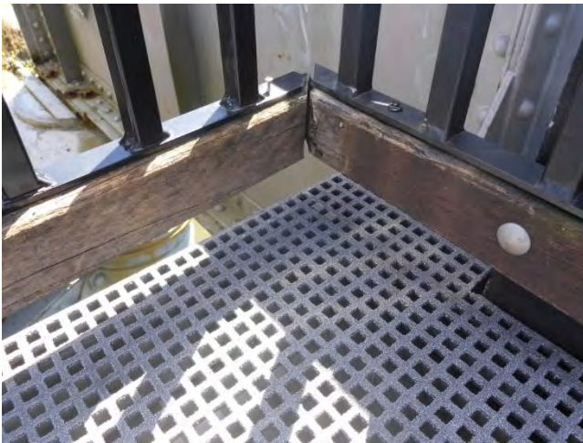
Photo 80 Connector plates not installed toe boards
