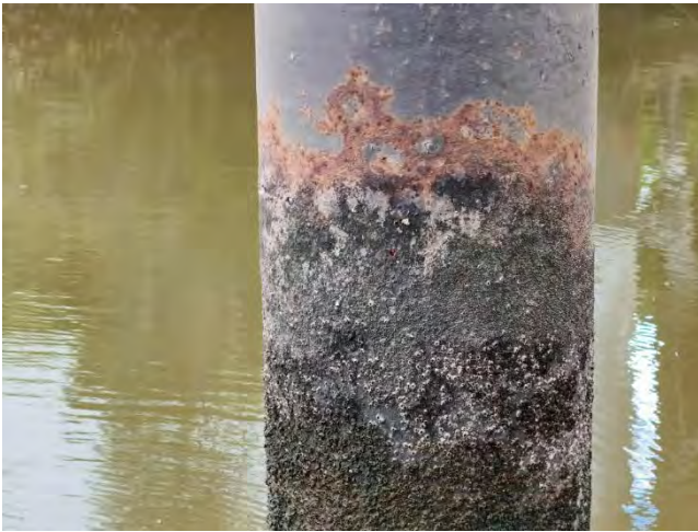
Photo 17 Pier 5 surface corrosion in tidal zone
