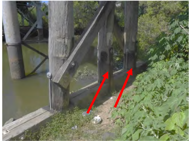
Photo 10 Base plates from the piers to timber footing exhibiting surface corrosion
