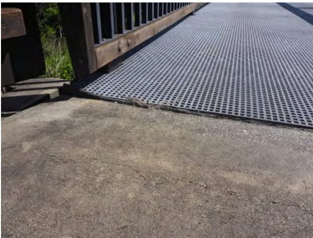
Photo 73 Approach 2 minor unevenness
