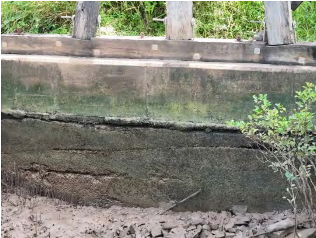
Photo 27 General view of pier 7 mass concrete footing, poor compaction typical
