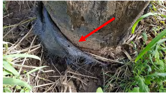
Figure 112: Example of weed matting found on some timber piers. Note the soil built-up in between the fabric and the timber (Converge 2022).
