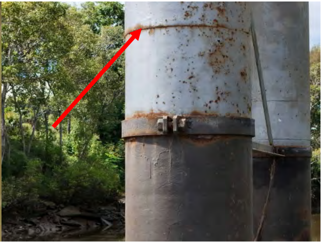
Photo 18 Pier 5 corrosion staining at welds and pitting corrosion in tidal zone
